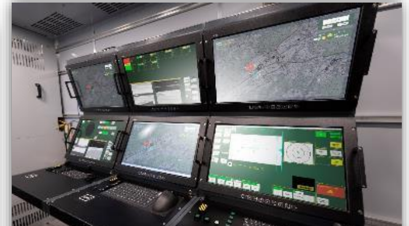
INTEGRATED COMMAND & CONTROL SYSTEMS
